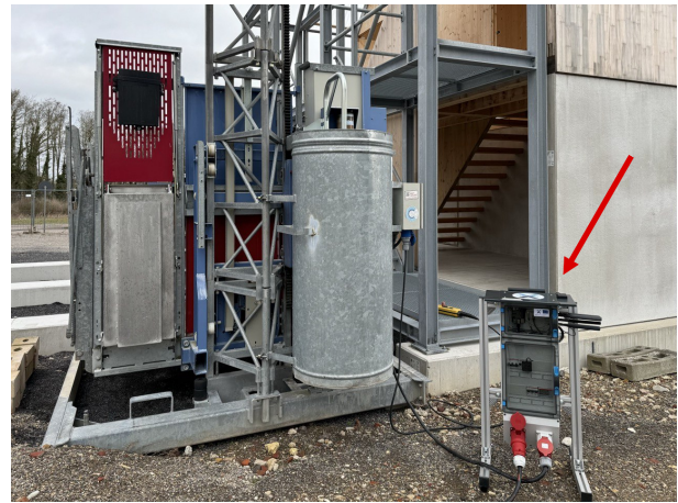
Figure 9: Experimental setup for the power measurement with the Meter-X device connected to the material lift.
