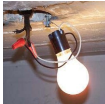
Figure 2: A makeshift lightbulb with exposed wiring
