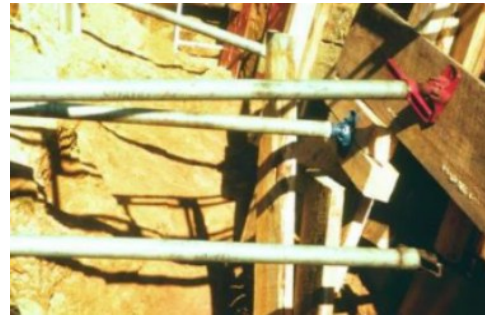
Figure 3: Improper shoring in a trench
