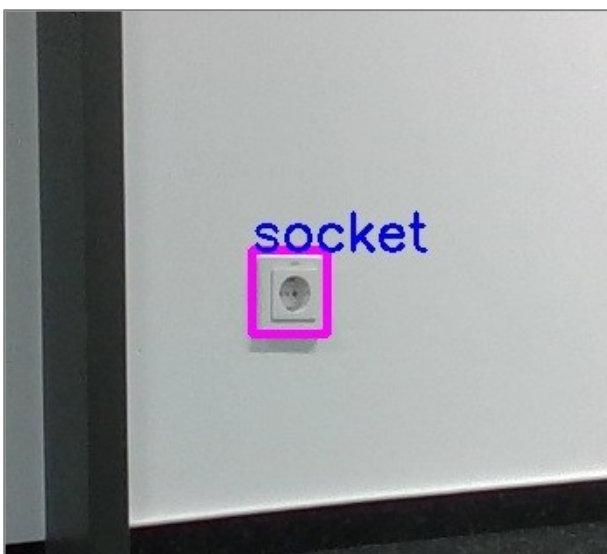
Figure 8: Image of the electrical outlet automatically captured during the visual inspection task
