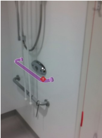
Figure 4: Deviation in the location of the toilet room grab rail
