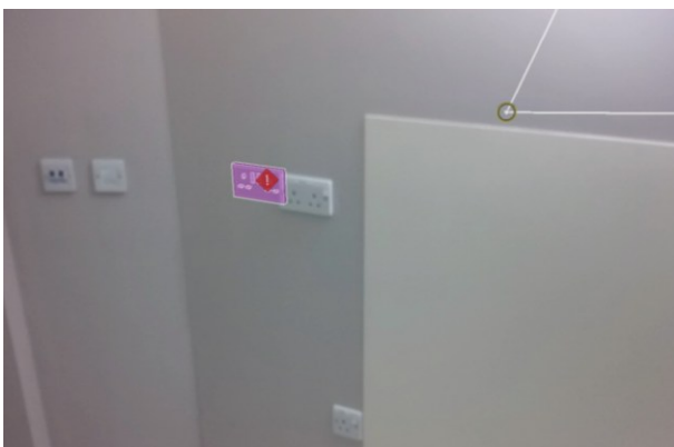
Figure 5: Deviation in the location of the electrical outlet
