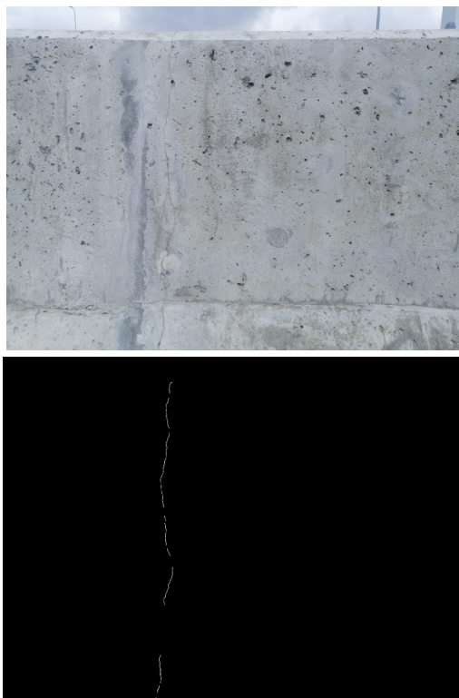
Figure 3: Example of image and corresponding segmentation mask (white pixels - crack, black pixels - background)
